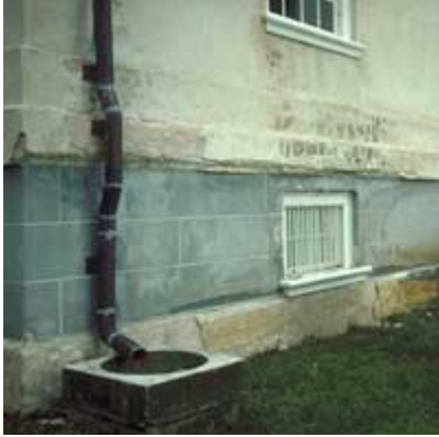
The damage to this stucco appears to be caused by moisture infiltration. Photo: NPS files.
