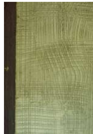
The final finish coat will be applied to this scratch coat. Photo: NPS files.
