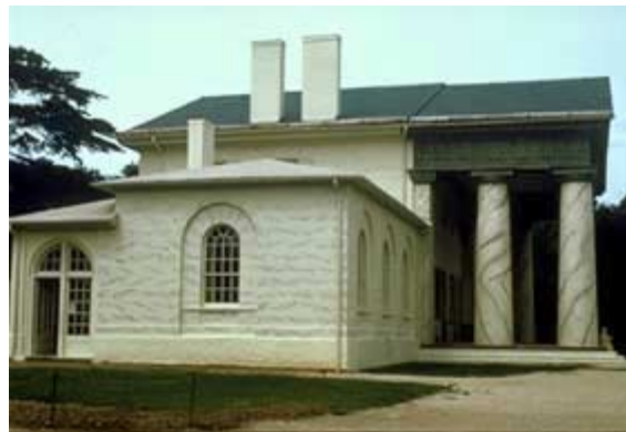
The stucco finish on Arlington House, Arlington, Virginia, was marbled in the 1850s, approximately 30 years after it was built. Photo: NPS files.
